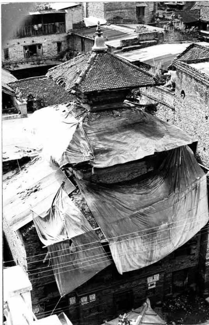
The Agache seen from the southeast, after emergency assistance by K.V.P.T. including tarpaulins on roof to protect building from monsoon rain, Spring 1992.
