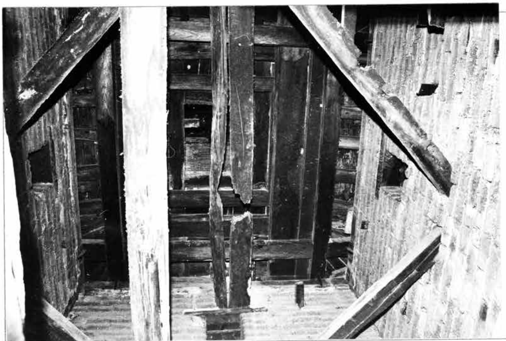
Below : Inside timber structure of upper pagoda showing damaged tie in center and corner bracing, perhaps added in 19th c. reconstruction. August 1993.
